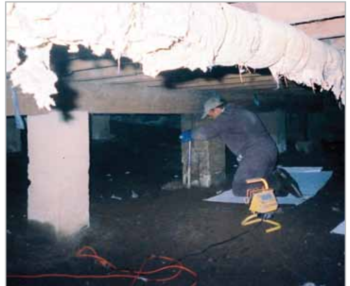
Miller and crew installed 40 baited ATBS stations under the structure. Within the first 30 days Miller had hits on 22 of the 40 stations.
