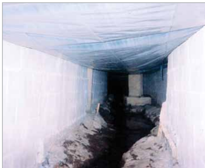
Brown Exterminating completely covered the crawl space floor and sealed the stream with plastic and an EPA-approved absorbent material to keep particles from entering the stream.
